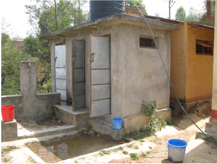
The 2 “connected” but non-functioning toilet buildings
